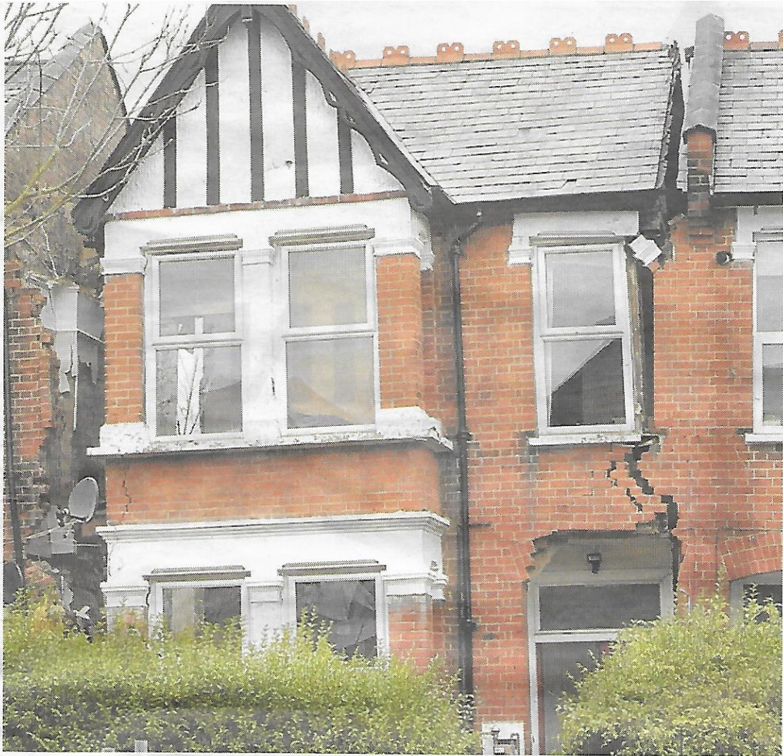
Ruined: Shoddy building work caused the Edwardian terraced home to crack and collapse PICTURE: CASCADE
